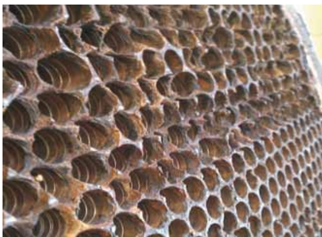
▲ Figure 2. Galvanic corrosion can occur in an HVAC system with a mild-steel tubesheet and copper tubes; this corrosion can be severe (bottom).
