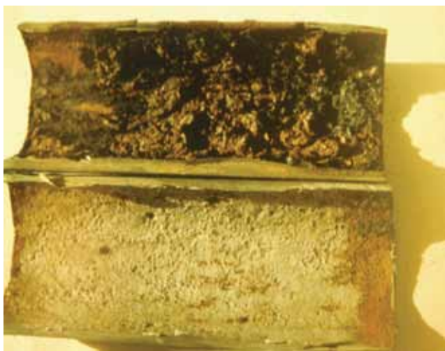
▲ Figure 3. Significant corrosion can occur in mild-steel piping prior to startup. This 1.5-in. pipe experienced severe corrosion within three months of installation (top); the bottom image shows the pipe after it was cleaned.
