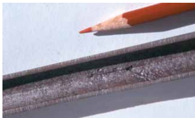
▲ Figure 4. Incomplete welds in mild-steel pipe foster corrosion, and can eventually lead to leaks.
