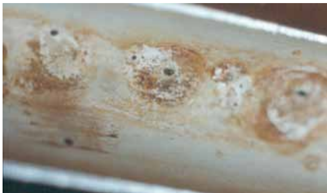
▲ Figure 6. MIC corrosion occurs in untreated stainless steel condenser tubes. The black spots are perforations due to corrosive bacteria.
